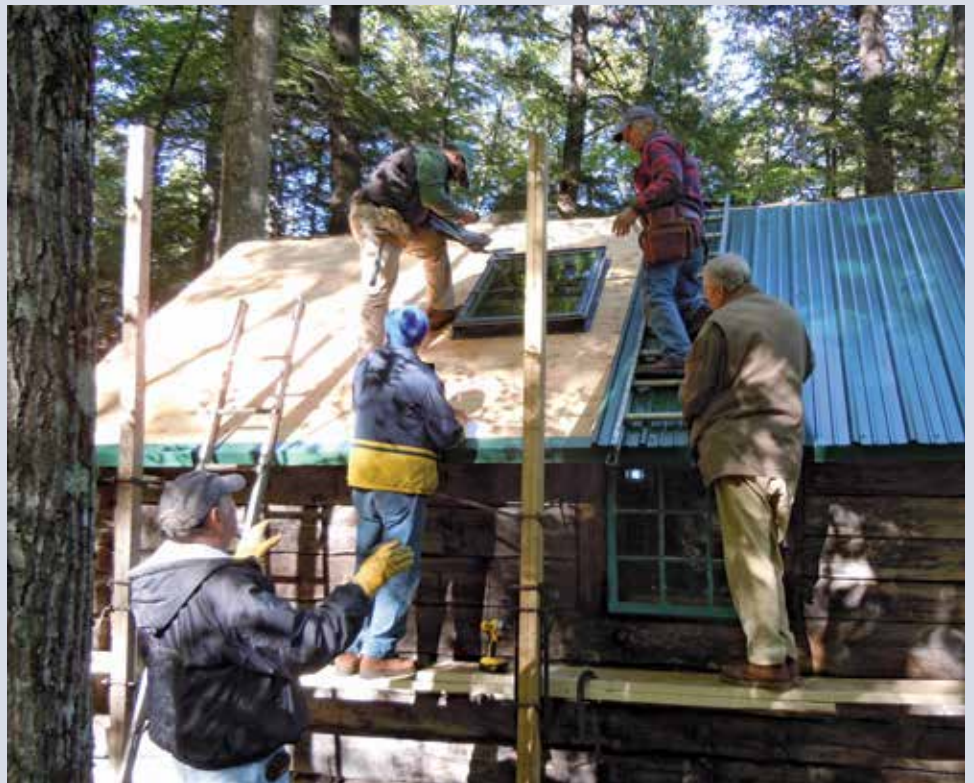
Members of the Meredith Rotary Club hard at work replacing the cabin roof
